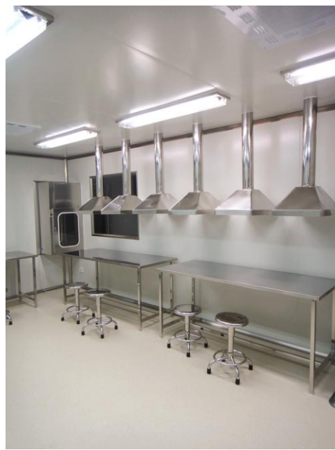
洁净车间/Clean Room
