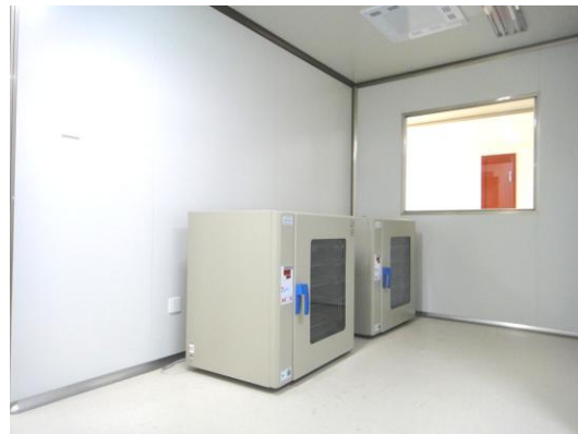
洁净车间/Clean Room
