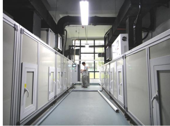
十万级空调系统/Air Conditioning System 1
