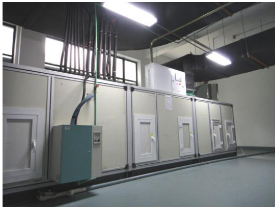
万级空调系统/Air Conditioning System 2
