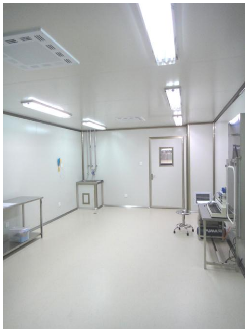
洁净车间/Clean Room
